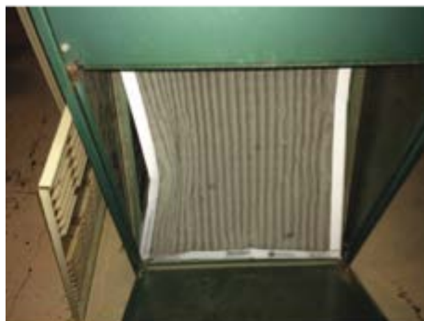
Damaged & clogged filters EPA-402-F-09-002
