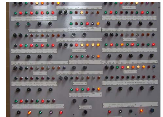
Control panels that are designed so that lay people can identify an alert (progressive) (flickr.com)
