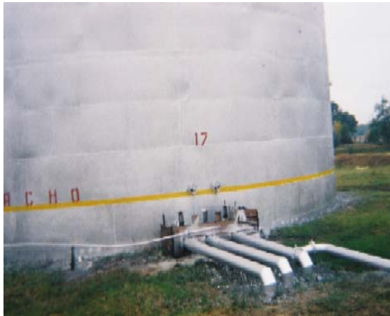
Picture 3: Flat bottomed tank with loamy ground and earth walls secondary containment
