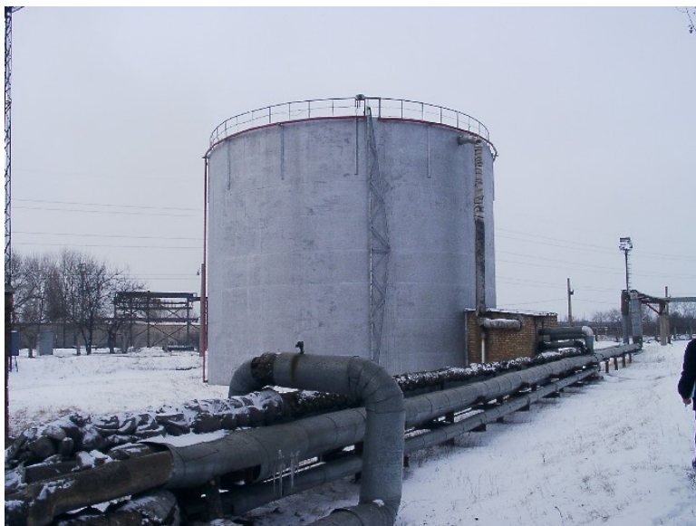
Picture 12: Masut - Tank
