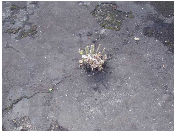
Picture 19: Destroyed tight surface, by plants
