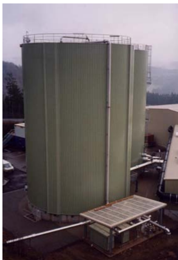
Figure 12 Digestion plant for bio-waste
